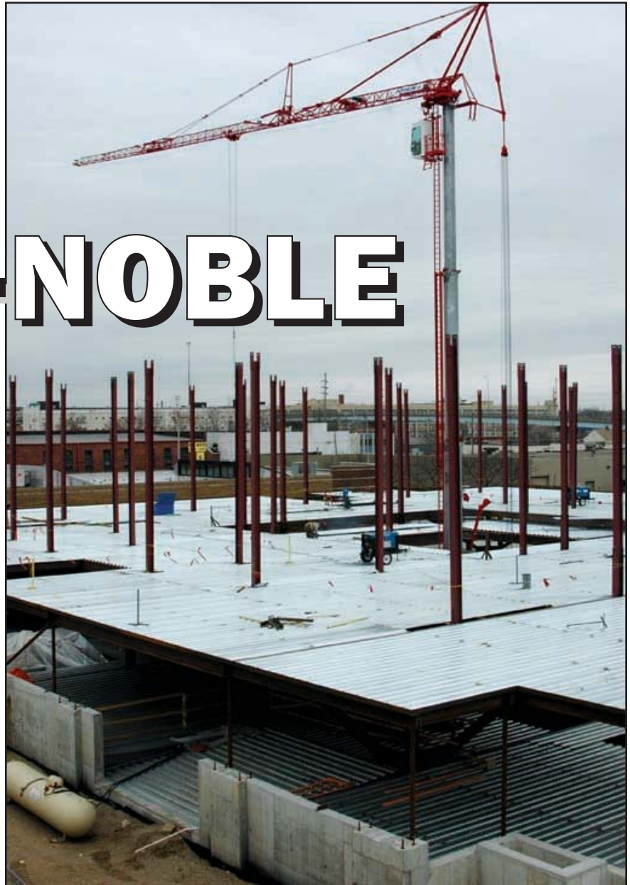
▲ The Maxwell condominium project is being built in the 500 block of East Ohio Street by Kosene & Kosene Development. It will feature upper-level residential units and street-level commercial space.
