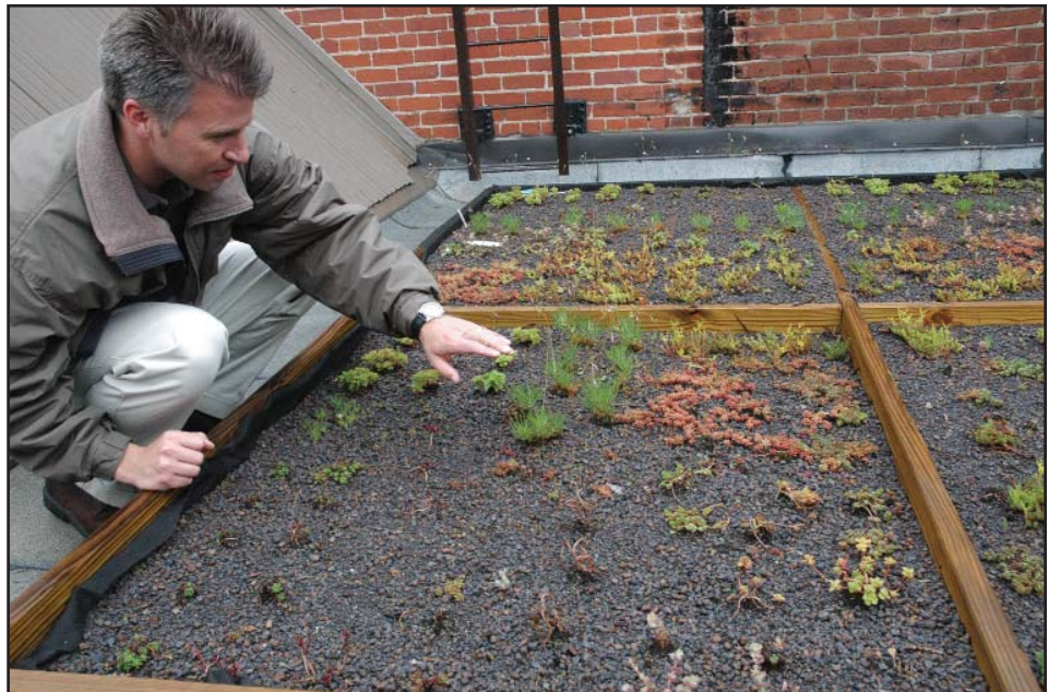
Craig Flandermeyer inspects the garden which has applications as roofing for flat-roofed structures such as schools and “big-box” stores.
