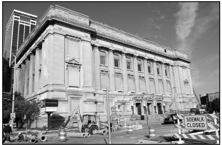
▲ The Old City Hall was listed on the National Register in 1974 and was documented for the Historic American Building Survey in 1981.
